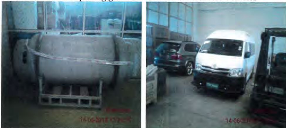
Picture 1: Ozone depleting gases not isolated from motor vehicles
