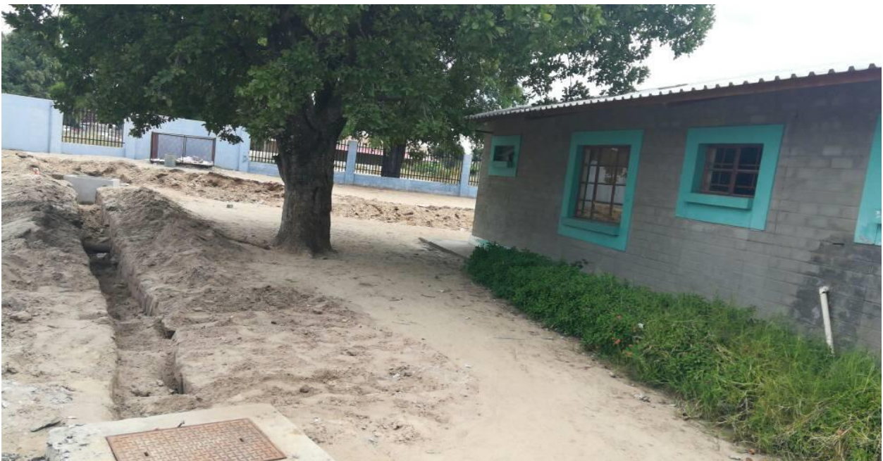
Fig.1 Sewer line at Ngweze Primary School in the Zambezi Region
