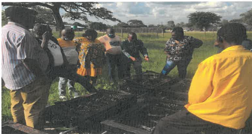
The picture above depicts vandalized and dilapidated water infrastructures in Sibbinda constituency, Zambezi region
