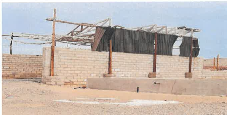
One of the structure that has been abandon at the Old De Beers sampling site
